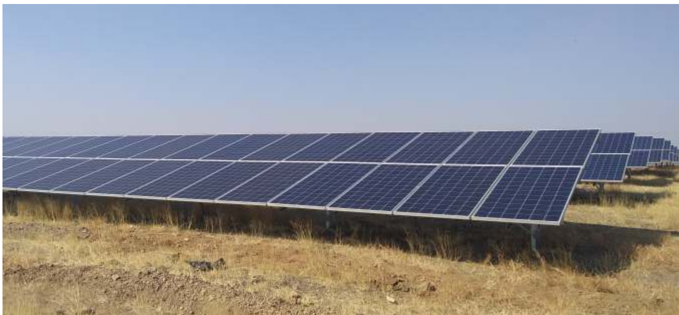
Axis Bank's 2 MW ground-mounted solar power project at Solapur, Maharashtra
